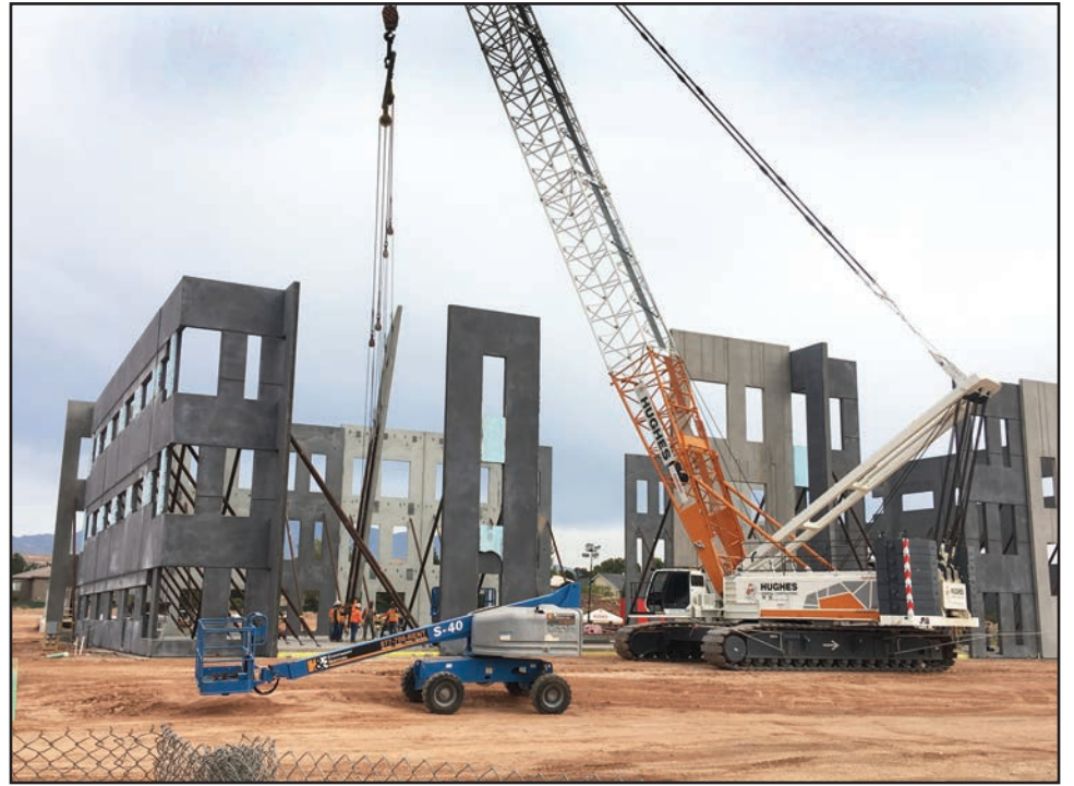
Hughes Construction used the tilt-up-panel construction method to expedite the construction of the Riverfront Medical Center in St. George to help doctors resolve clinic space shortages in the Southern Utah community.
