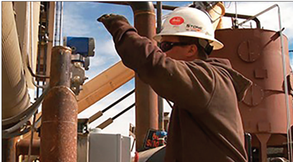
A worker takes a reading from a pressure gauge at Petroteq Energy's oil sands processing plant at Asphalt Ridge near Vernal. The company is extracting bitumen from Uintah County's vast oil sands deposits in a process it says is the cleanest and most efficient anywhere. Petroteq Energy Inc. photo.
