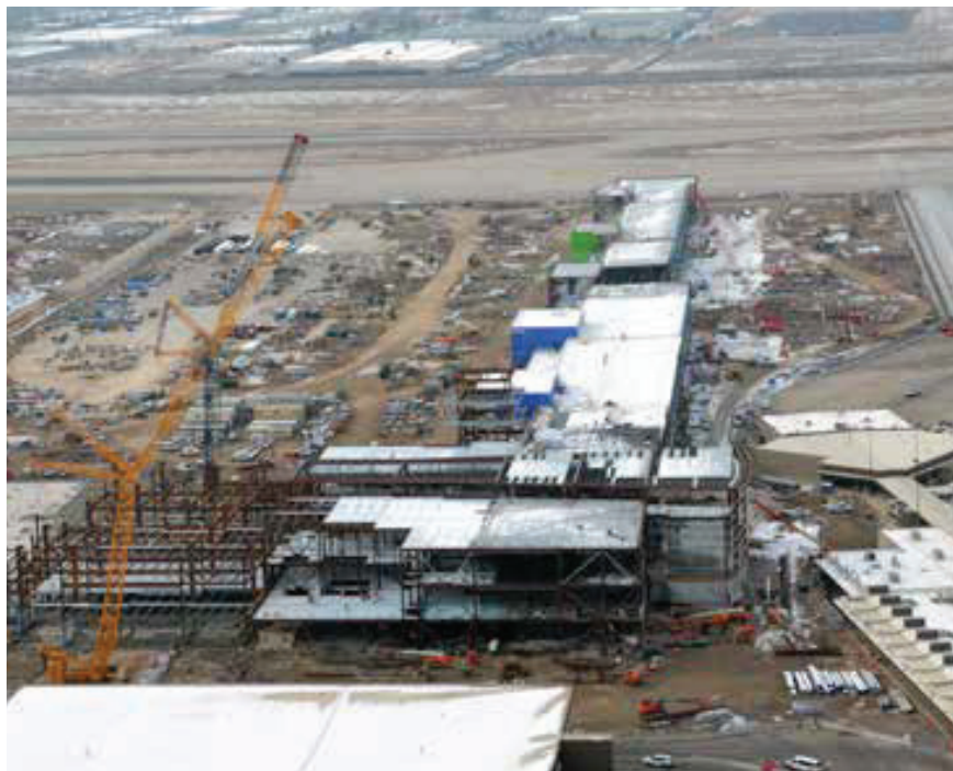
Aerial view of progress on the new South Concourse West building at The New SLC as of February 2018. The first phase of the Airport Redevelopment Program is expected to open in 2020.
