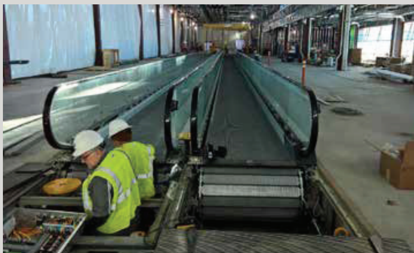
Teams install a moving walkway in the new terminal as part of the Airport Redevelopment Program. An estimated 63% of trades performing work on the project are from Utah firms.
