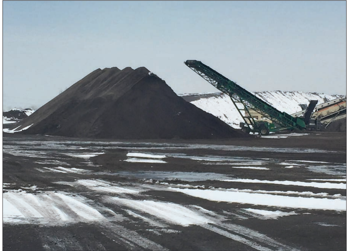
Anderson Geneva, the company redeveloping the site of the old Geneva Steel plant in Vineyard, has set up a major removal and recycling operation for the 750,000 cubic yards of concrete that must be dealt with before construction goes forward on the @geneva master-planned community. The company said it has removed 200,000 cubic yards of material to date and that it will take about three more years to complete the job.
