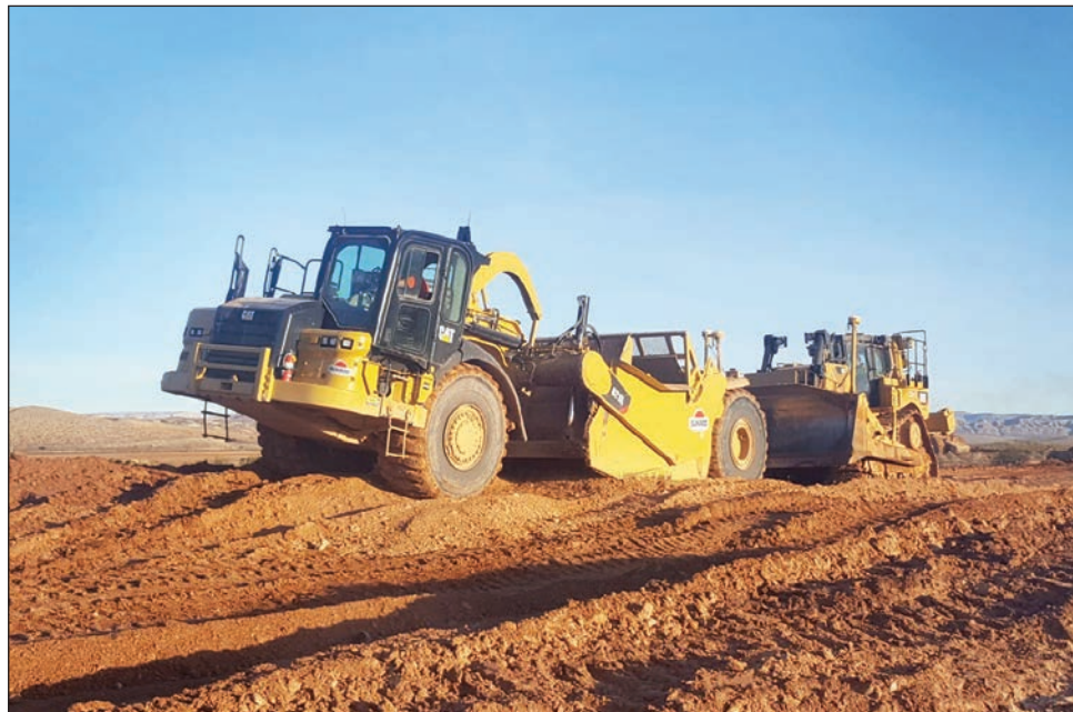
Heavy equipment from Southern Utah's Sunroc Construction has begun building roads, homesites and pads for retail businesses at the location of a recently announced master-planned community in St. George. To be called Desert Color, the project will consist of a commercial district, recreational facilities, a resort and up to 10,000 residences. (G. Lane Photography. St. George)
