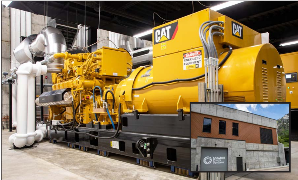
One of three massive Cat-powered generators sits ready for use in the Snowbird Power Systems electricity generating station in Little Cottonwood Canyon. The station gives the resort the ability to fulfill 100 percent of its power demand.
