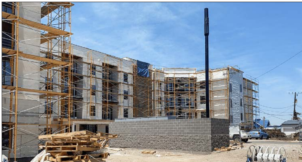
Builders are working overtime around Utah to create homes to ease the state's "unhealthy" housing shortage. That includes constructing multiple family units like the Capital Homes Apartments being built by Kier Construction in Salt Lake City. Photo courtesy of Kier Construction.
