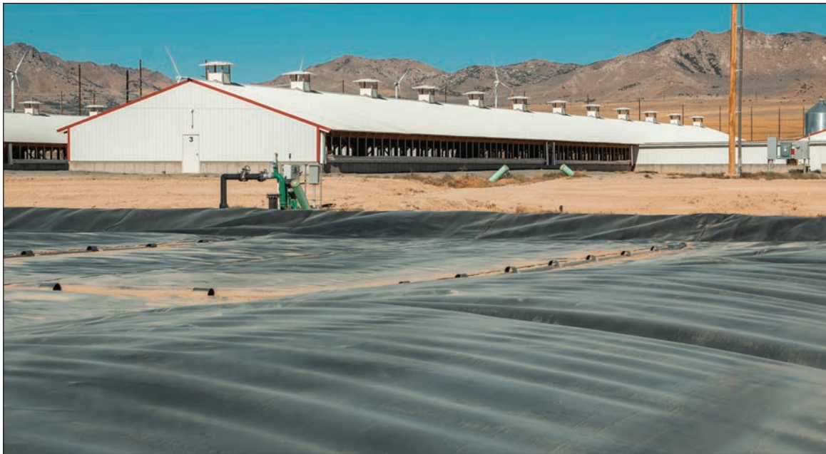
An anaerobic digester, part of the process of turning waste from hog farming operations in Beaver County into renewable natural gas, is shown on a farm near Milford. Dominion Energy and Smithfield Foods Inc. have launched the project on 26 farms in a cooperative effort to reduce the carbon footprint of protein-raising operations.
